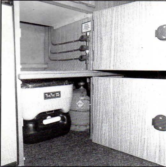
Three gas isolator taps are plumbed in line, and there's a home for two gas bottles and the standard loo
