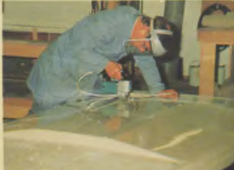
The aperture for a roof vent is cut before the hightop is mounted on the vehicle.
